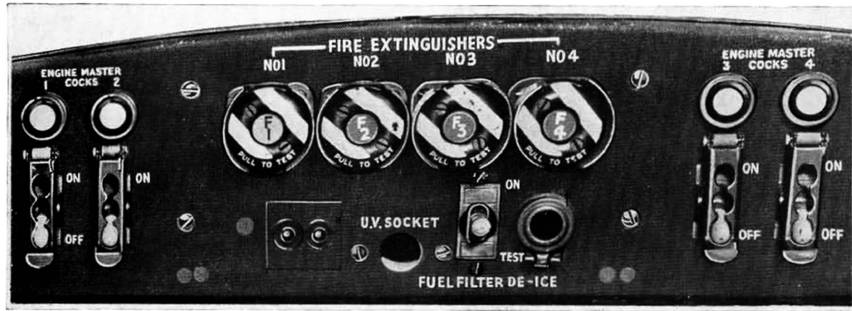
Fig. 29 Engine fire-extinguisher controls
