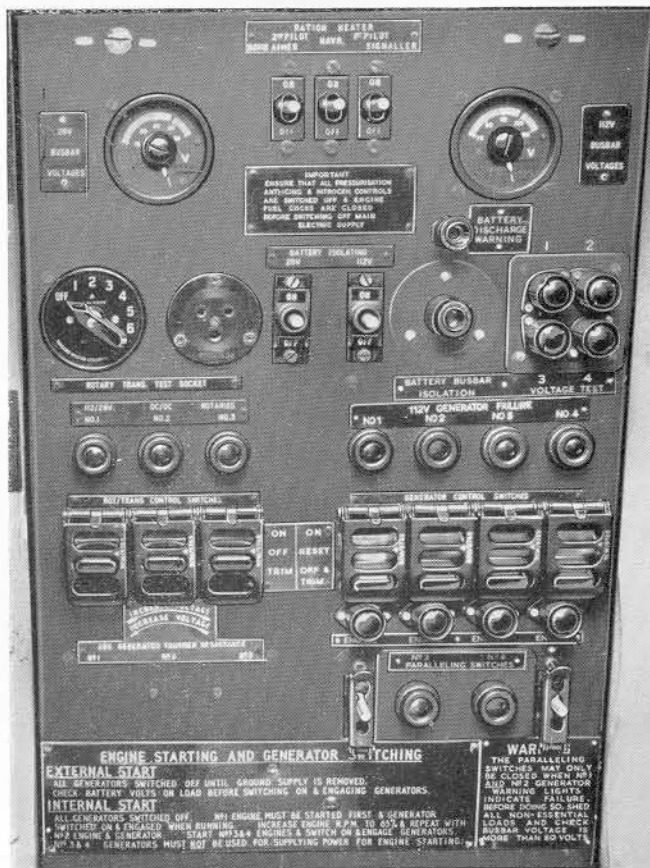
Fig 3 DC Control Panel
